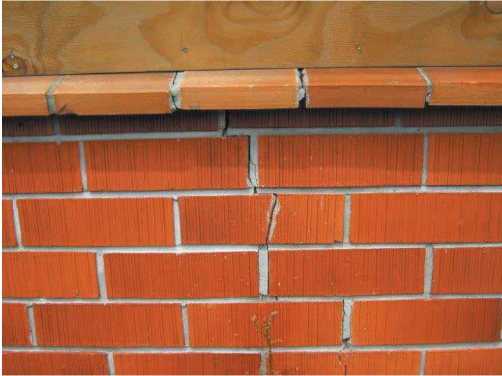
Image 3: Vertical split bricks and mortar
