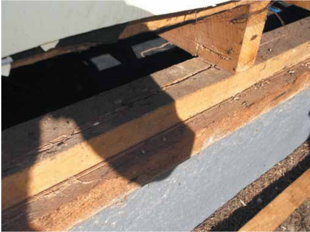
Image 6: Joists notched over bearer. Bearer remains fixed to beam
