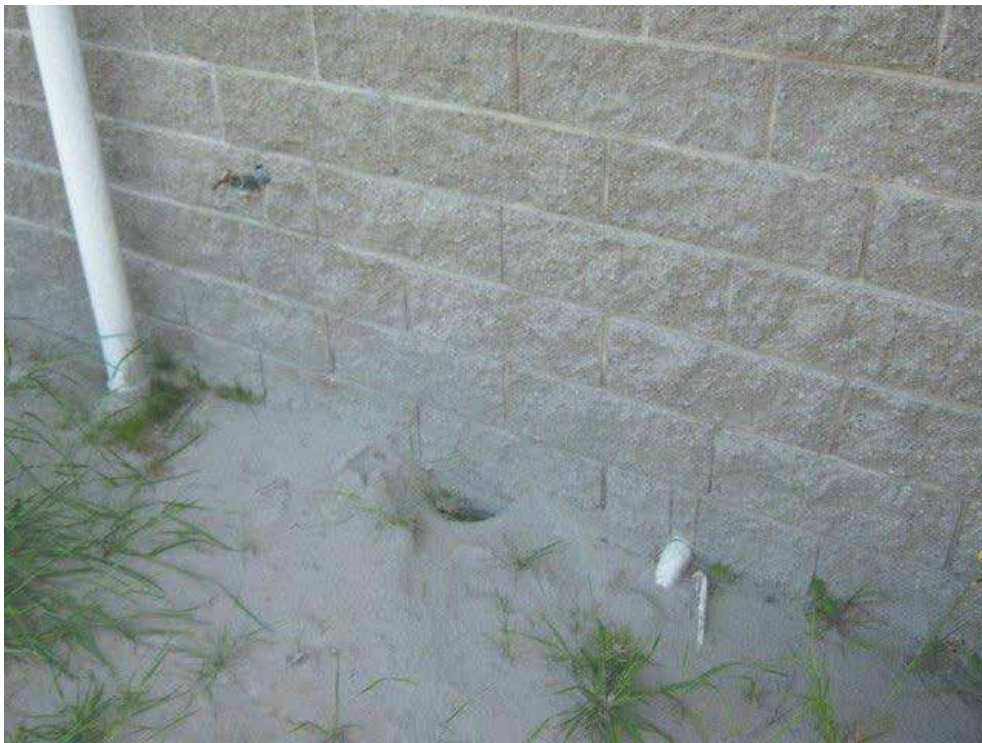
Image 1: Liquefaction ejecta potentially entered weep holes in veneer around perimeter
