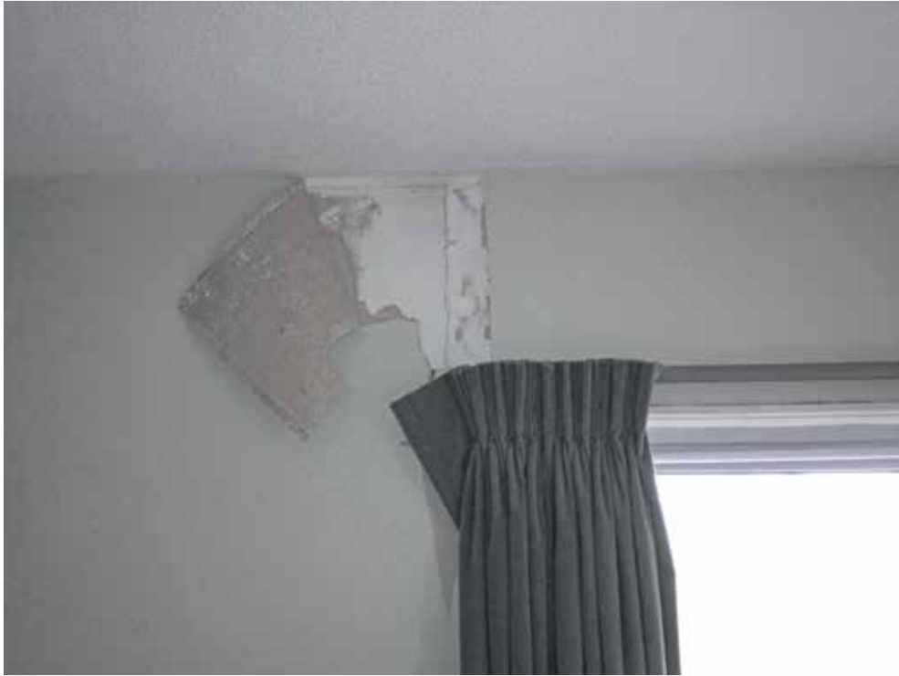
Image 9: Vertical cracks in plasterboard closed up after foundation relevel
