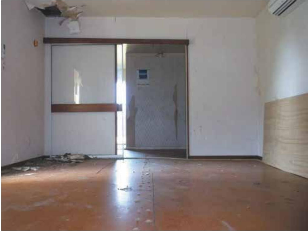
Image 4: Uneven floor settlement
