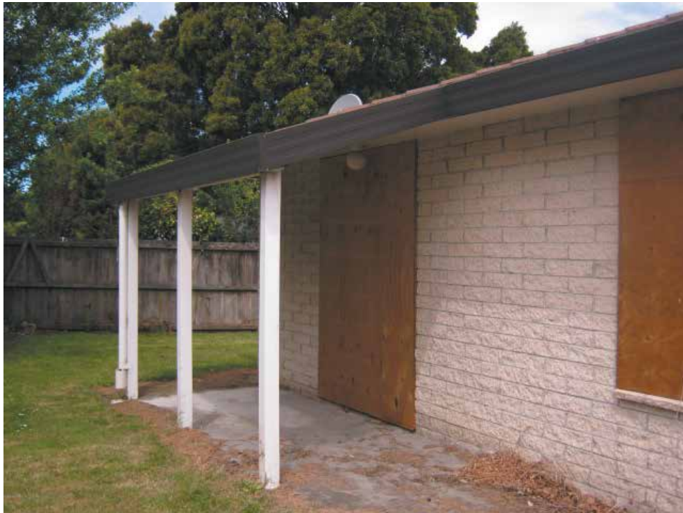
Image 1: Unit settled below ground level
