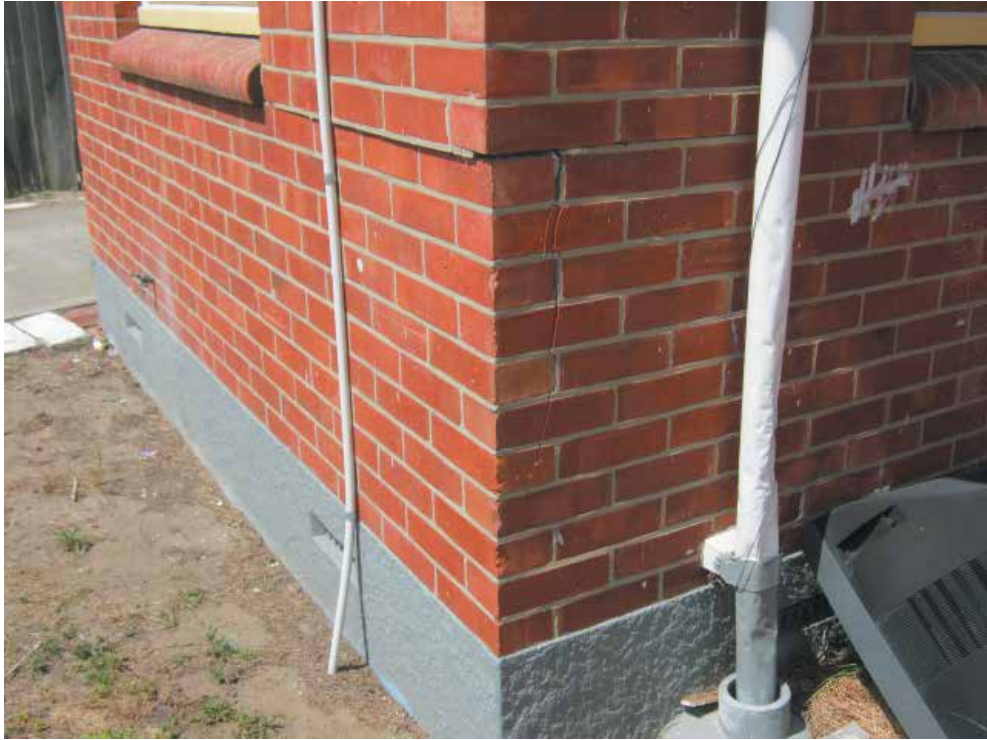
Image 2: Existing brick veneer. Horizontal displacement
