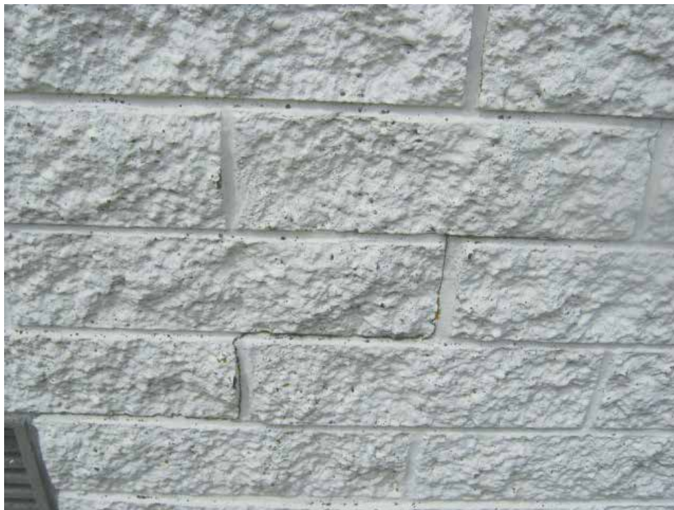
Image 1: Minor step cracking in veneer
