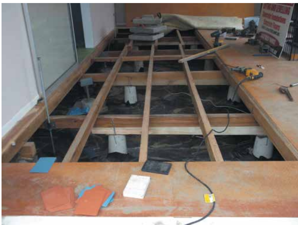
Image 10: Where lift was over 100 mm, piles were packed with an extra bearer spanning at least two piles
