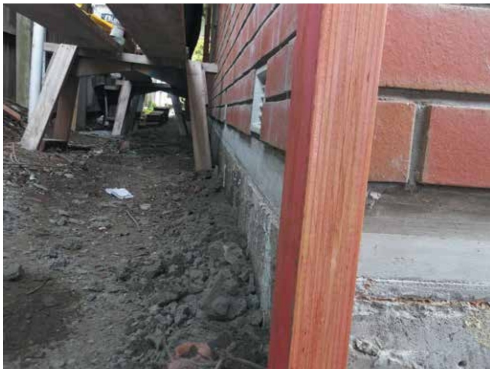
Image 13: Offset new cladding to allow foundation to be plastered in line with brick veneer
