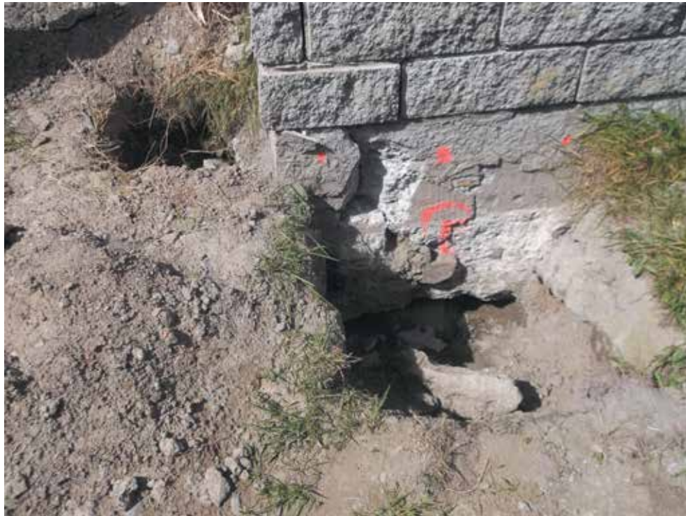
Image 11: Damage to foundation beam caused by bracket being installed too close to the corner. Foundation repairs were necessary to remedy
