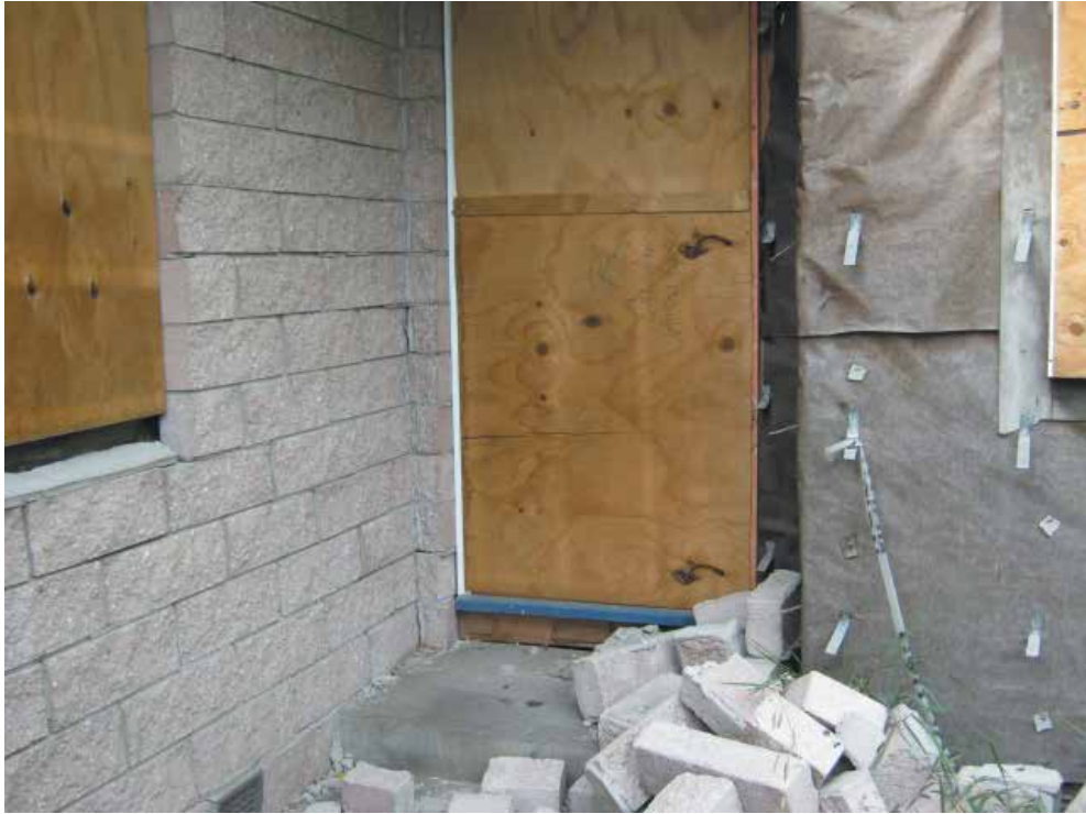
Image 4: Failed brick ties
