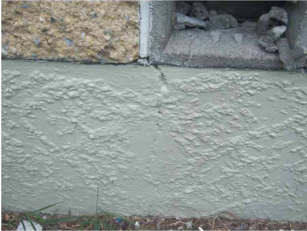
Image 4: Pre-existing foundation crack that appeared to have been repaired before the earthquakes
