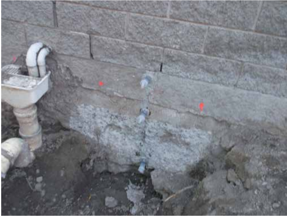
Image 9: Void fill under perimeter foundation beam and beneath concrete slab. New and existing cracks in foundation repaired with epoxy compound injection
