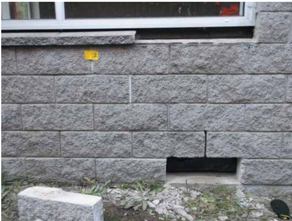
Image 11: Gap between sill block and window frame indicates separation between floor slab and foundation perimeter beam
