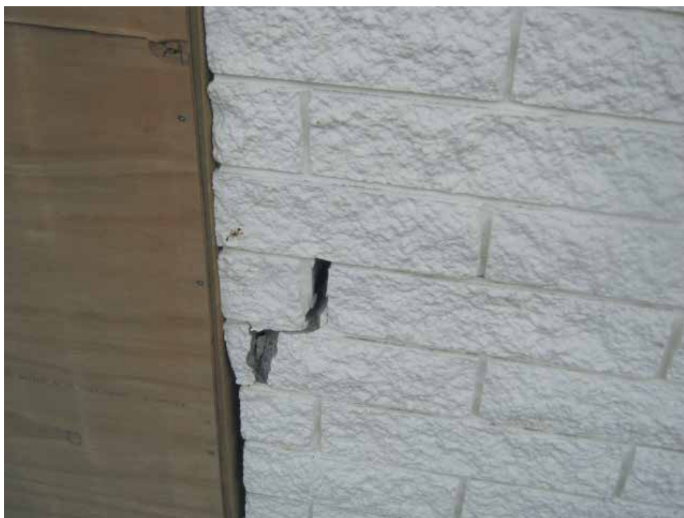
Image 1: Moderate brick veneer damage
