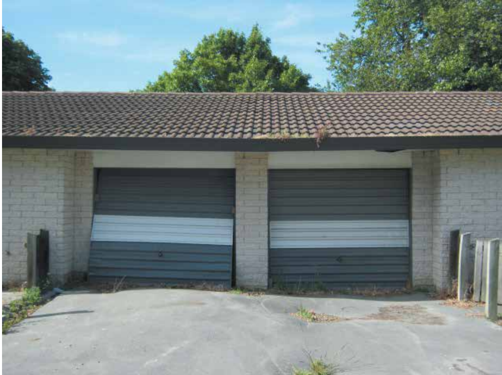
Image 3: Garage drive hump and sand boil
