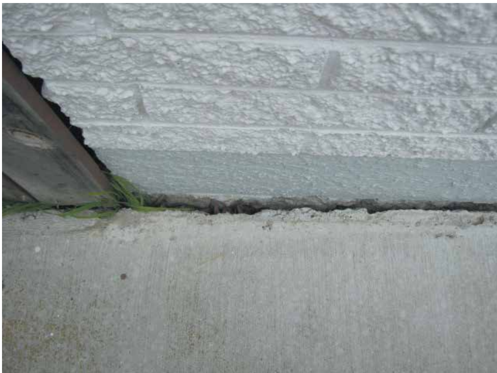
Image 3: Lateral spreading of hard surfaces
