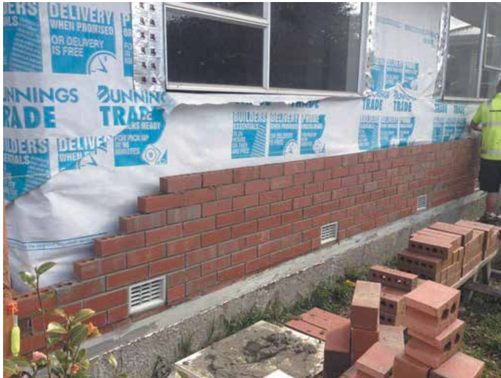
Image 12: Brick slithers laid to bring foundation level where a topping of more than 1:1 ratio required
