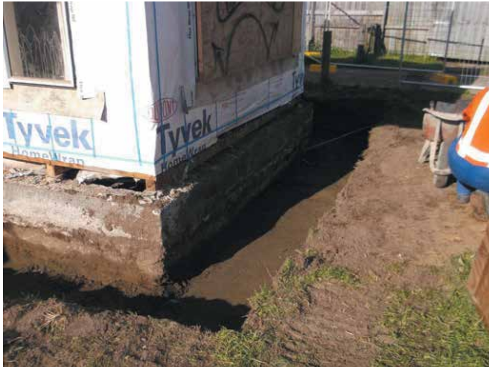
Image 5: With cladding removed, opportunity taken to insulate and wrap. Trench excavated around foundation perimeter for access to footing
