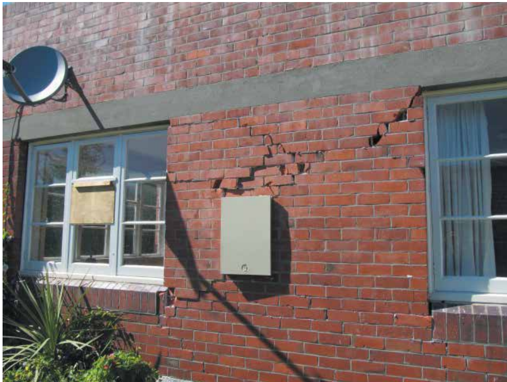
Image 4: Foundation settled at corners causing damage to veneer
