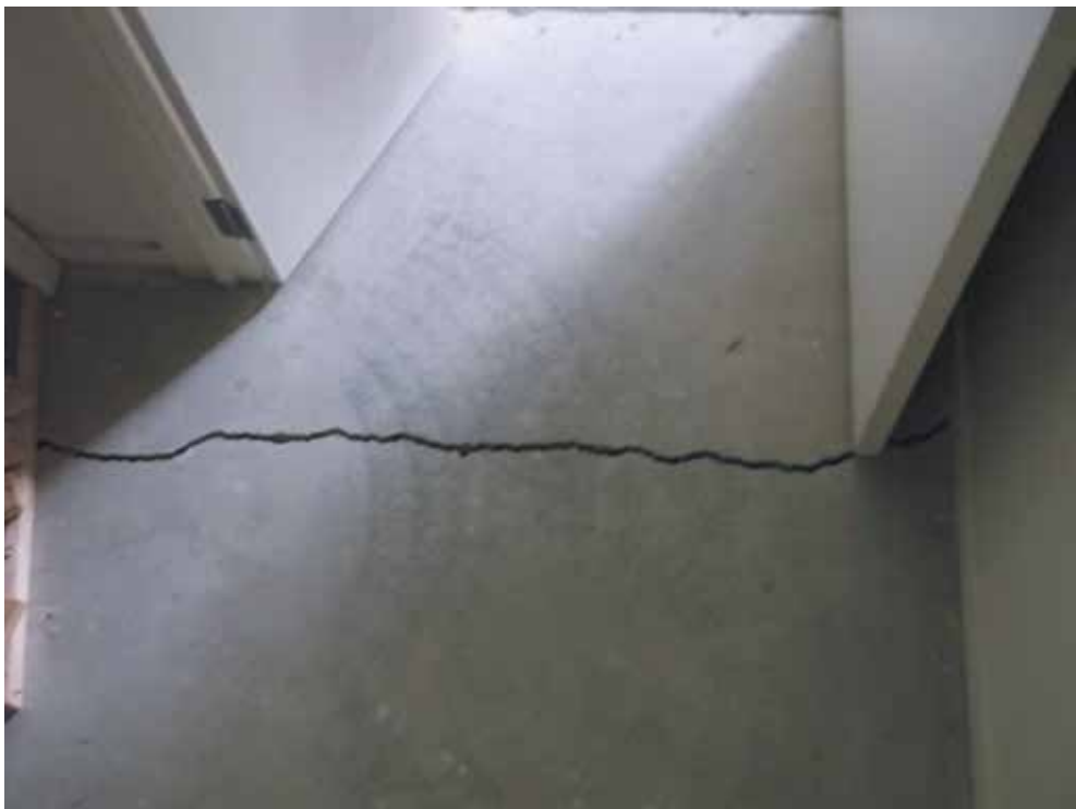
Image 3: Moderate slab crack of 8-15mm through width of floor
