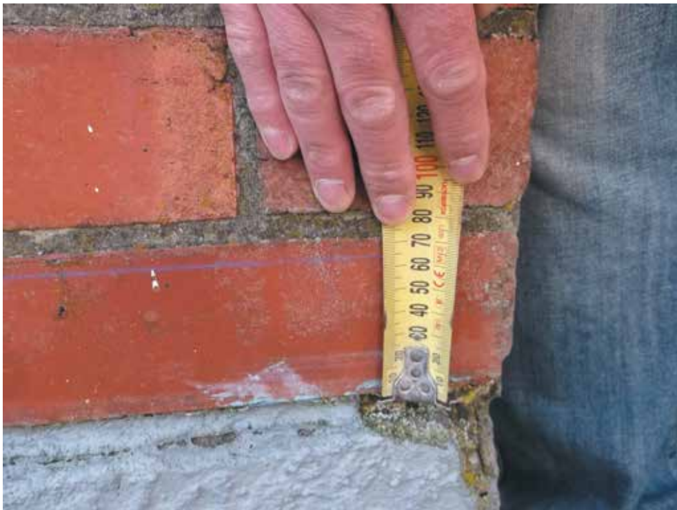
Image 1: 65mm vertical settlement at this corner
