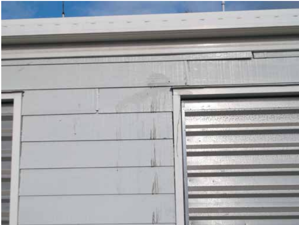
Image 1: Spreading of weatherboard cladding in the garage where foundation pulled in opposite directions
