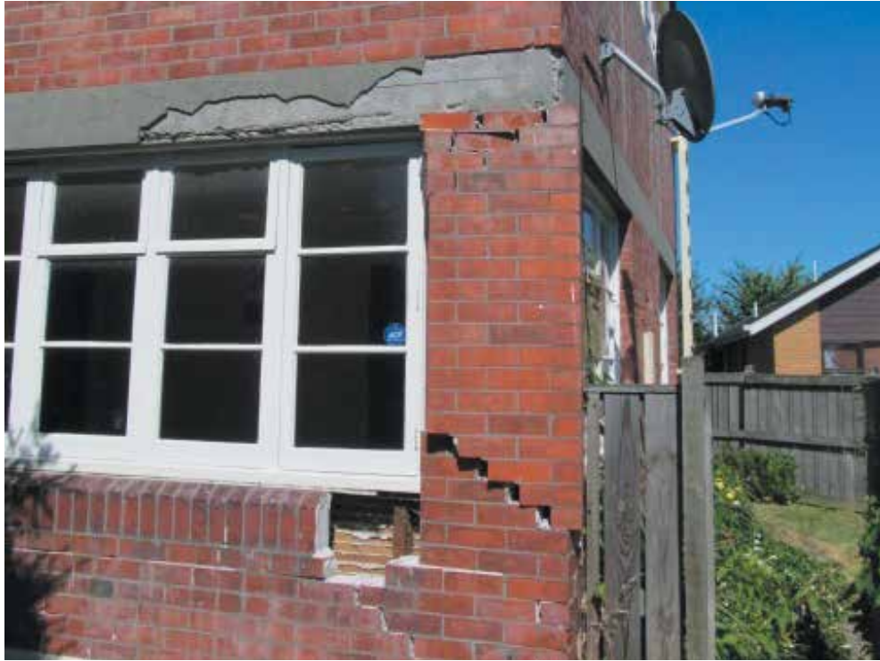
Image 3: Vertical and step cracking of bricks and mortar
