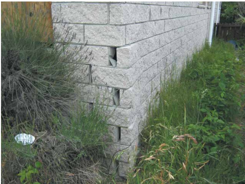
Image 3: Bricks dislodged, failed connection to framing
