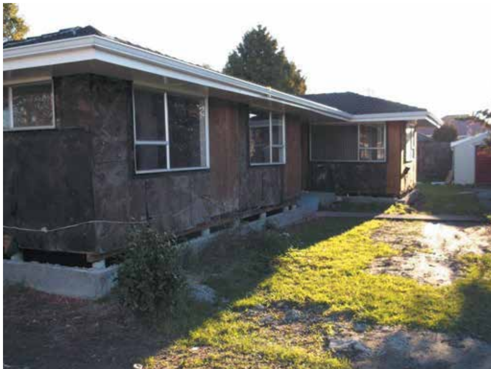
Image 6: Cladding removed. Opportunity taken to replace any worn insulation and new wrap installed
