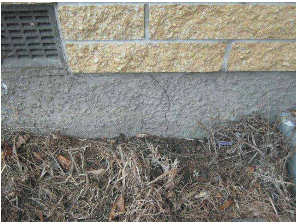
Image 3: Minor damage to foundation
