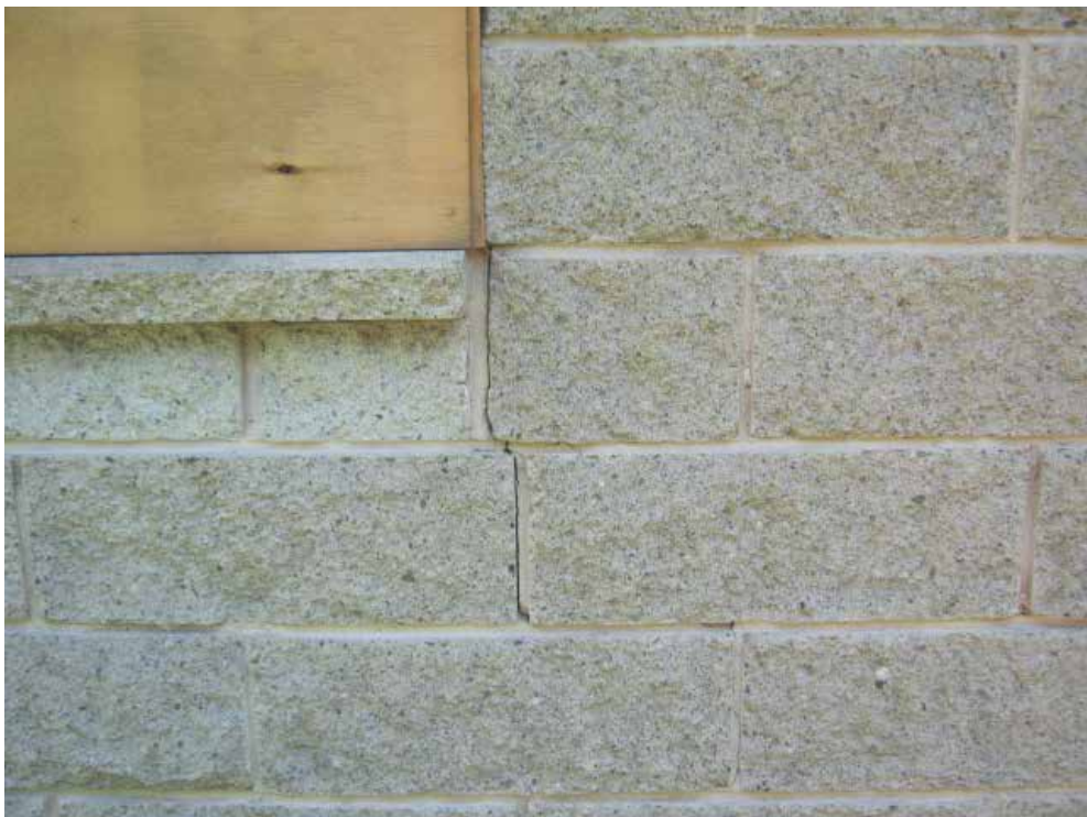
Image 3: Vertical cracks in veneer
