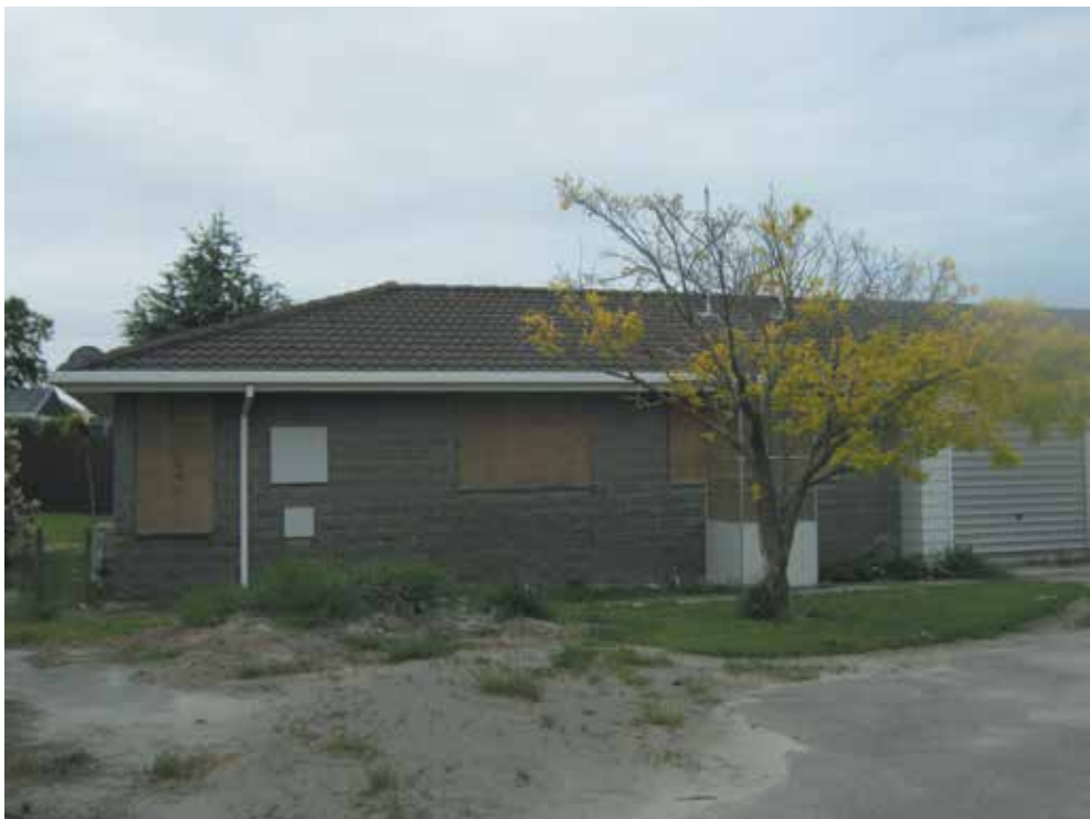
Image 5: Significant liquefaction ejection over half the site
