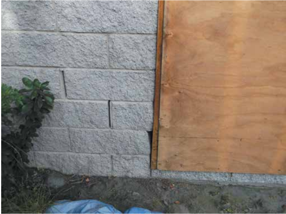
Image 2: Lateral spread of Summerhill Stone cladding caused by slippage on the foundation
