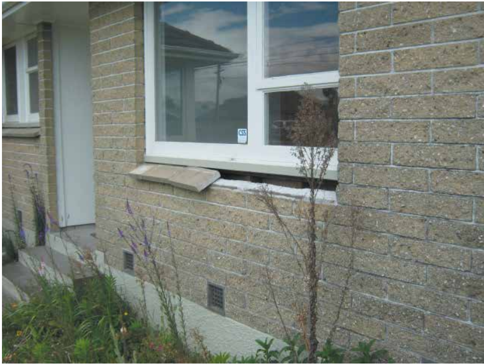
Image 2: Damage to brick veneer at windows
