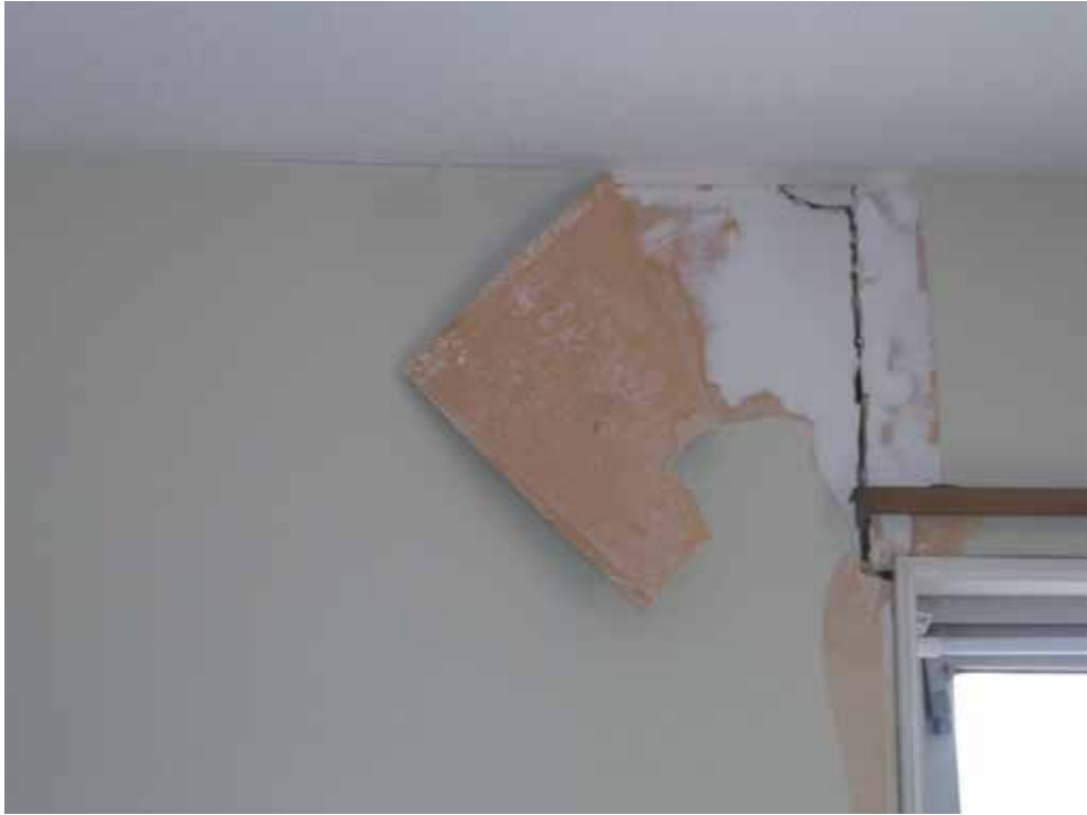
Image 4: Cracks at joints between plasterboard sheets from the corner of the opening
