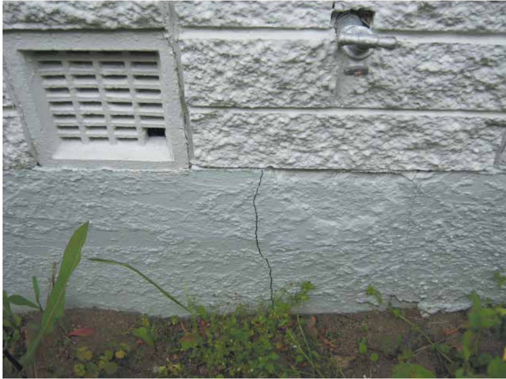
Image 4: Minor cracking to concrete perimeter foundation
