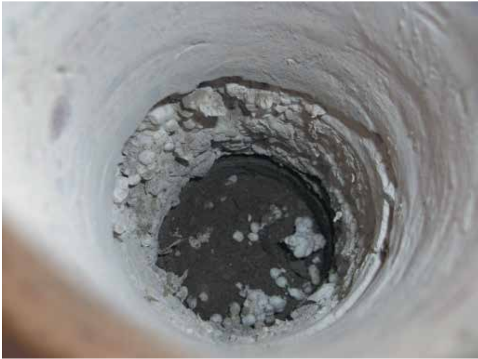
Image 6: Internal core holes drilled for void fill injection points and to release possible slab suction
