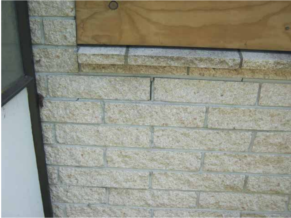
Image 4: Minor masonry veneer cracking
