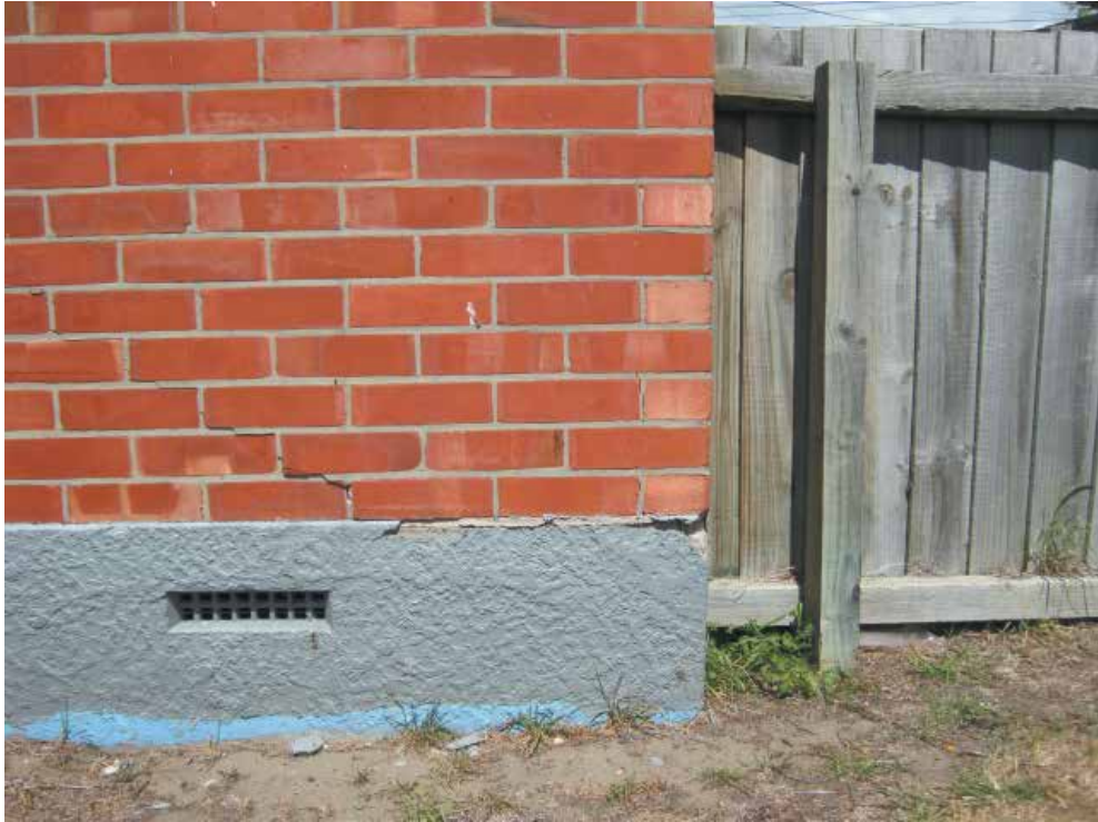
Image 3: Veneer damage and movement on foundation
