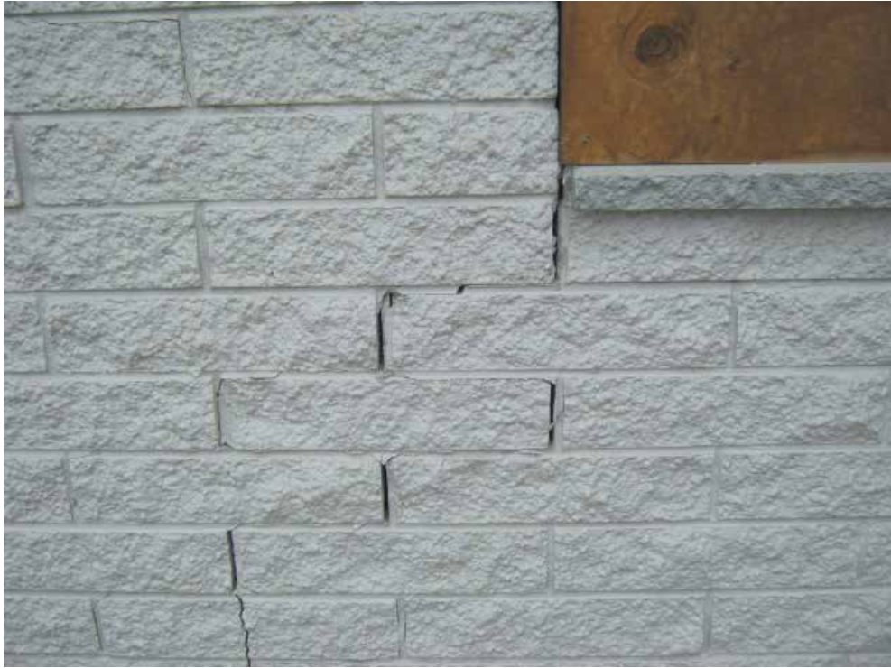
Image 2: Step cracking in mortar
