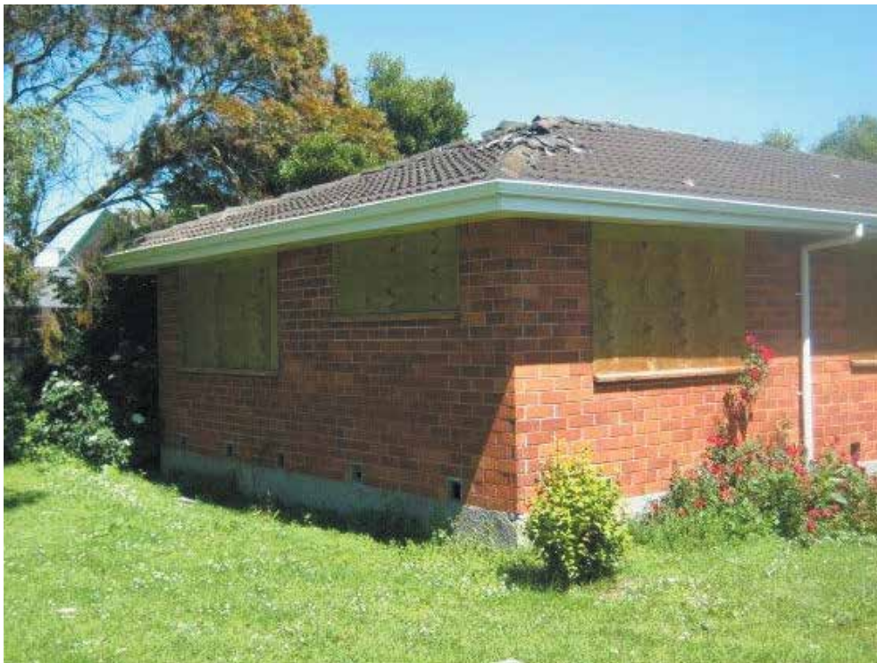
Image 1: Moderate damage to heavy weight roof
