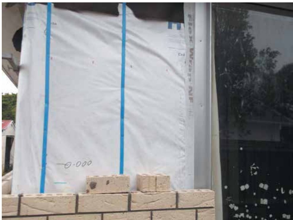
Image 12: Aluminium window flashings installed to provide cover for window at brick junction
