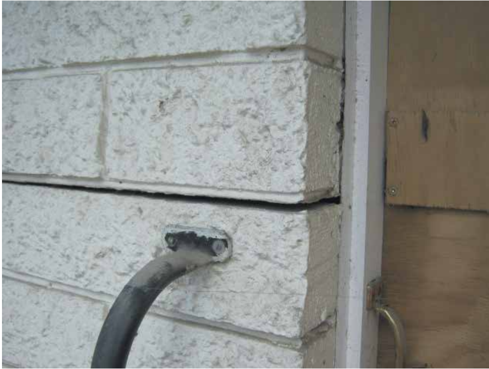
Image 2: Bond failure of the mortar allowing separation of brick courses under differential settlement of the foundation beneath
