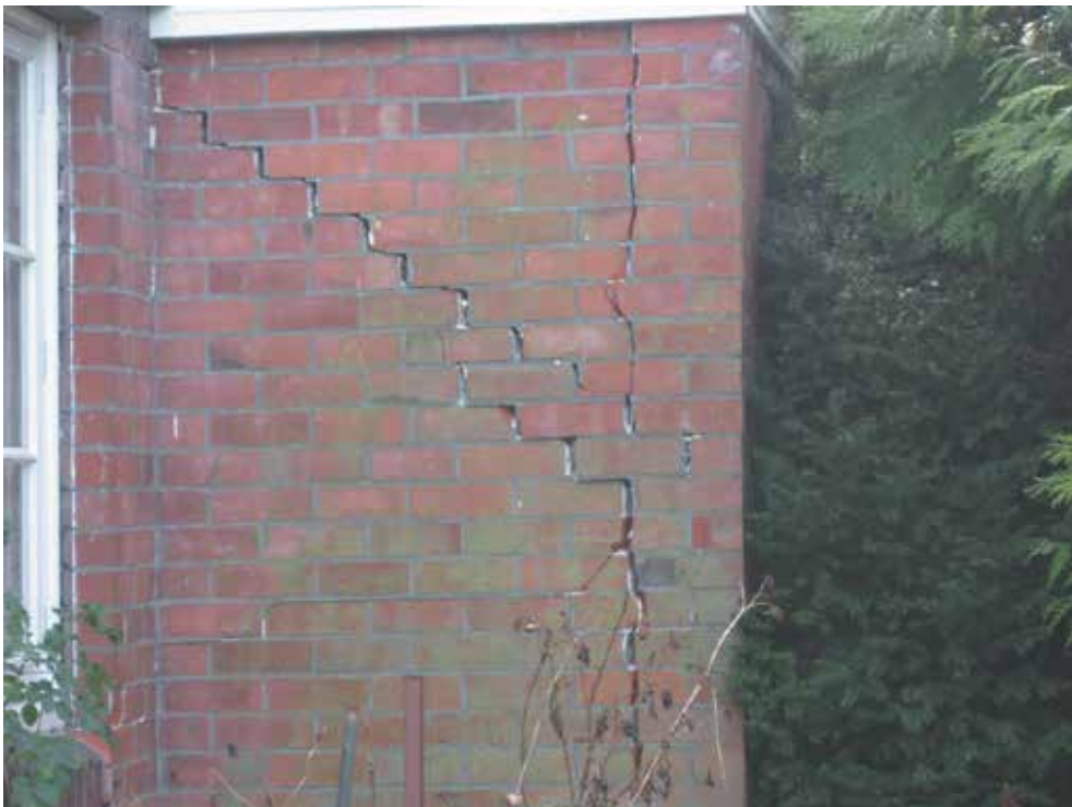
Image 2: Vertical and step cracking of bricks and mortar
