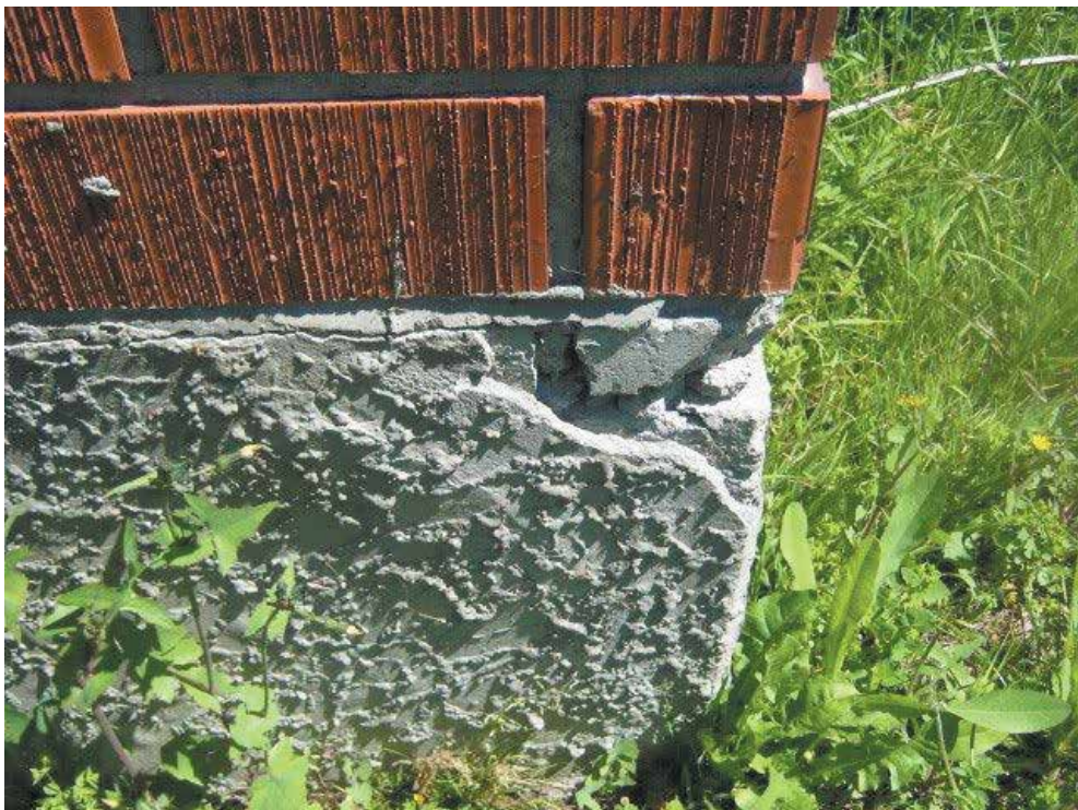
Image 5: Minor foundation damage
