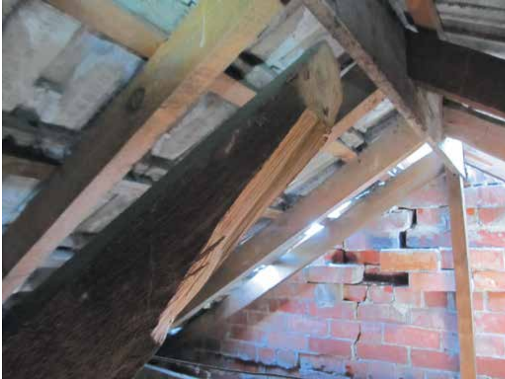
Image 1: Roof lost structural integrity
