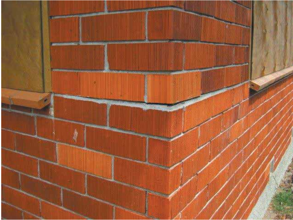
Image 4: Foundation has settled at corners causing damage to veneer
