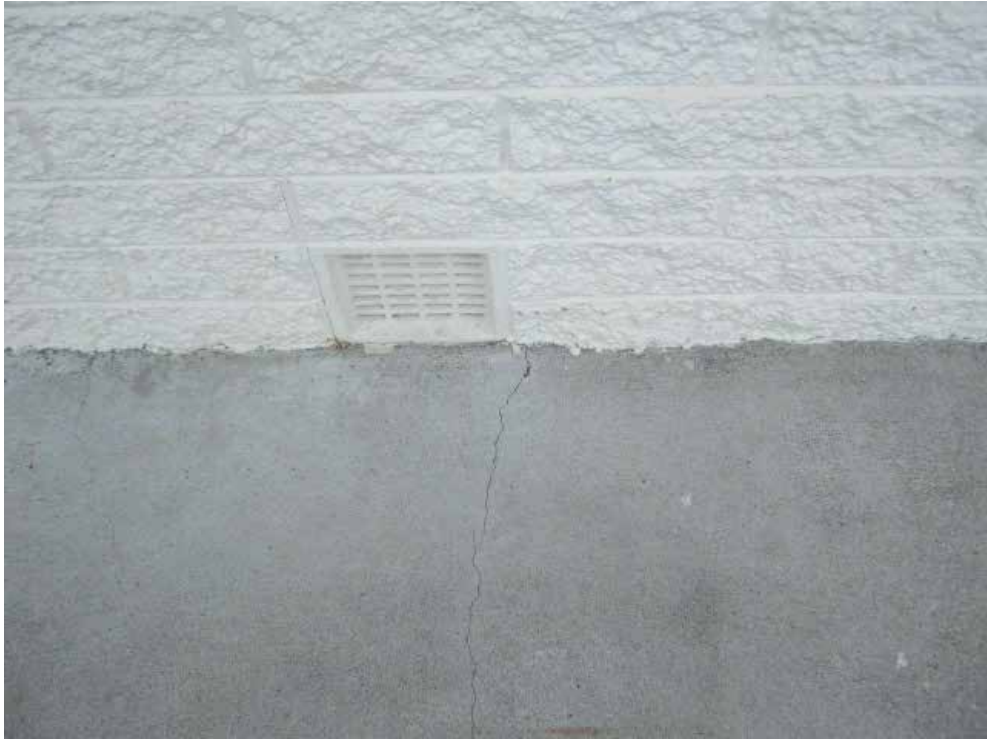
Image 2: Hairline crack in foundation
