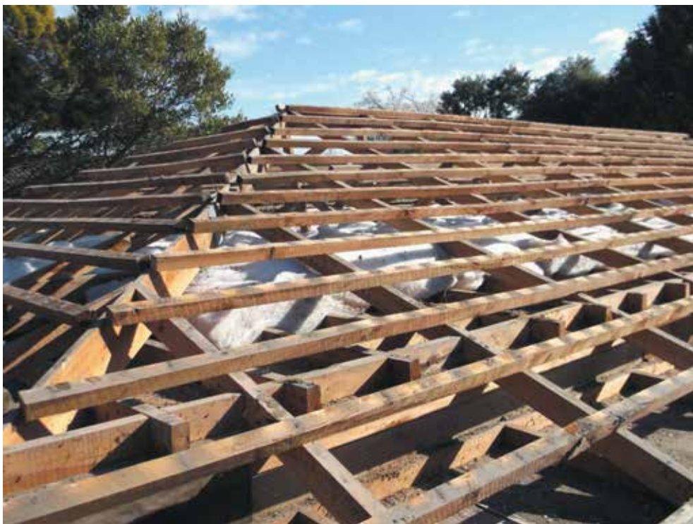
Image 9: Roofing removed. Opportunity taken to insulate areas not accessible from roof space
