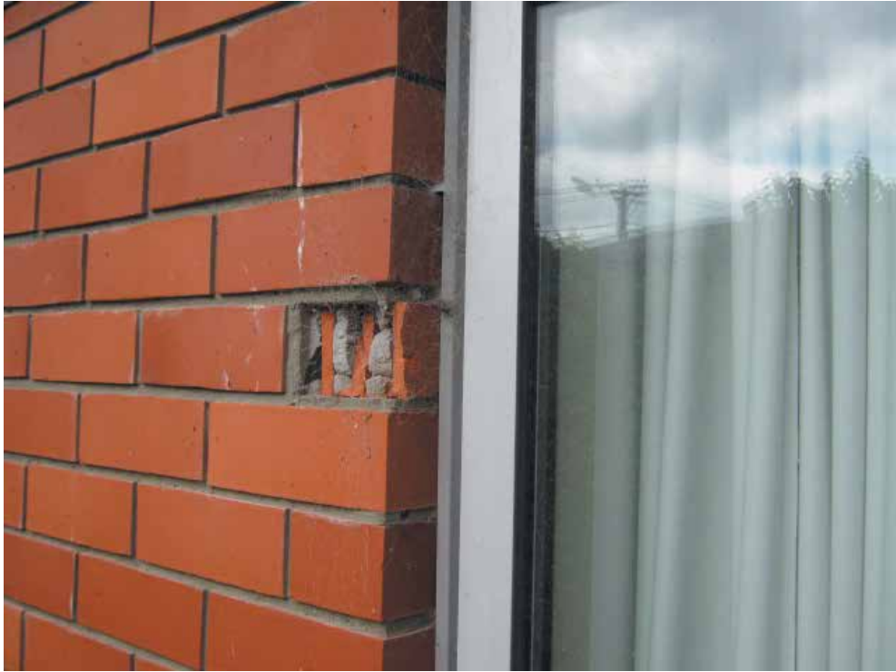
Image 2: Loose bricks, lost connection with brick ties
