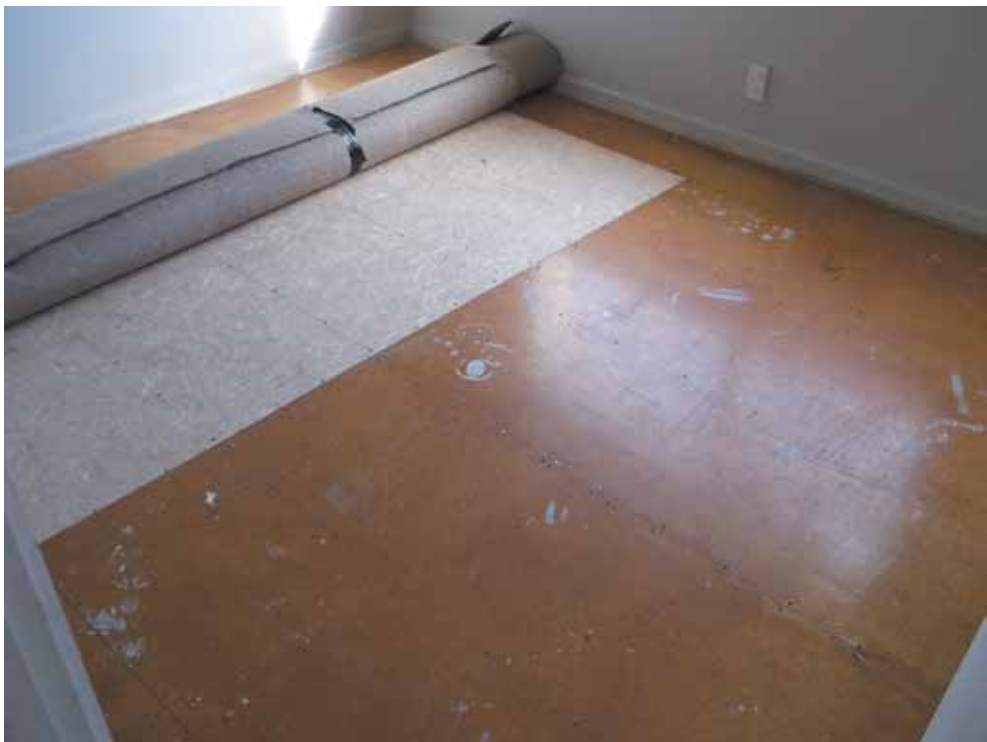
Image 7: Internal flooring replaced with original materials if available and fixed down using glue and screws
