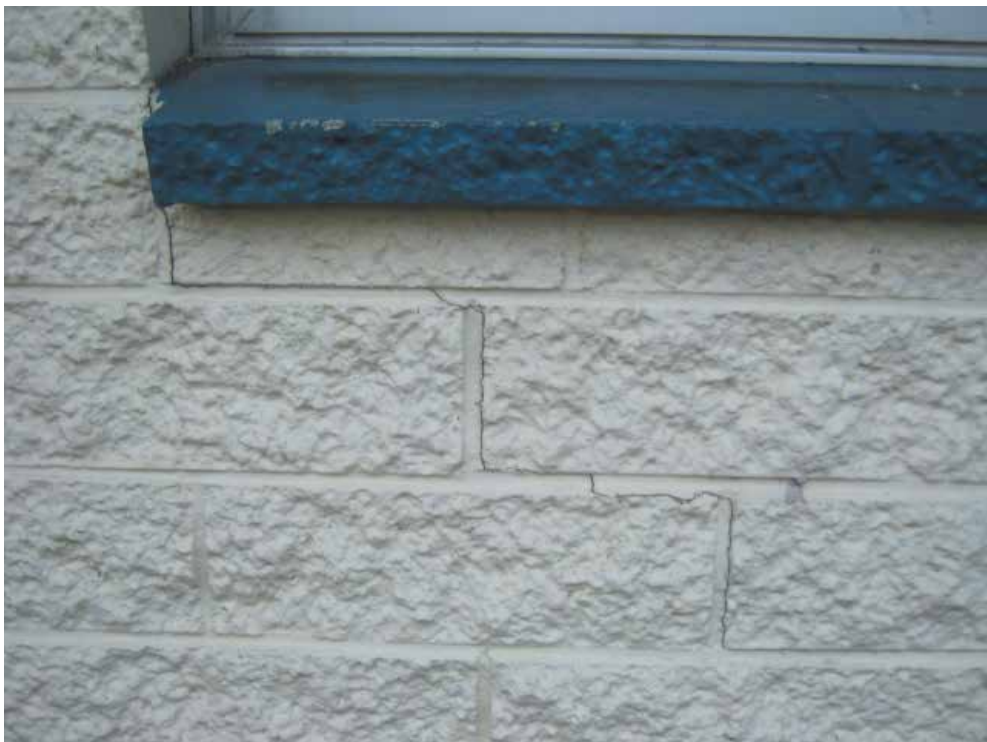
Image 3: Minor step cracking from window corners
