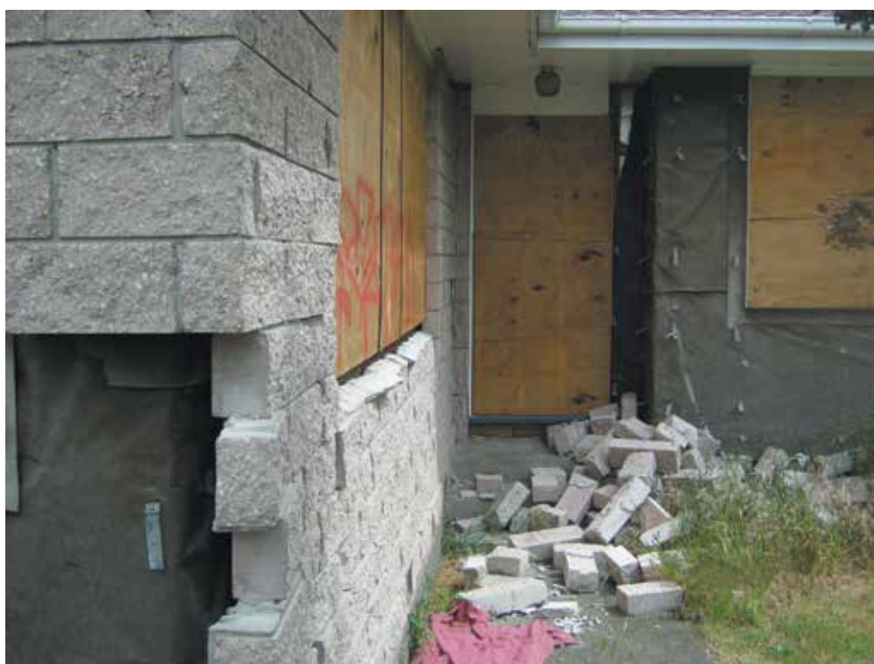
Image 1: Major veneer damage
