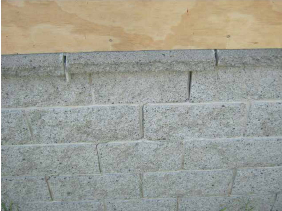
Image 4: Step cracking in mortar
