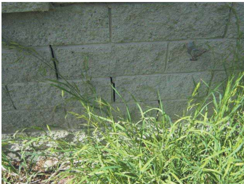
Image 3: Step cracks in mortar
