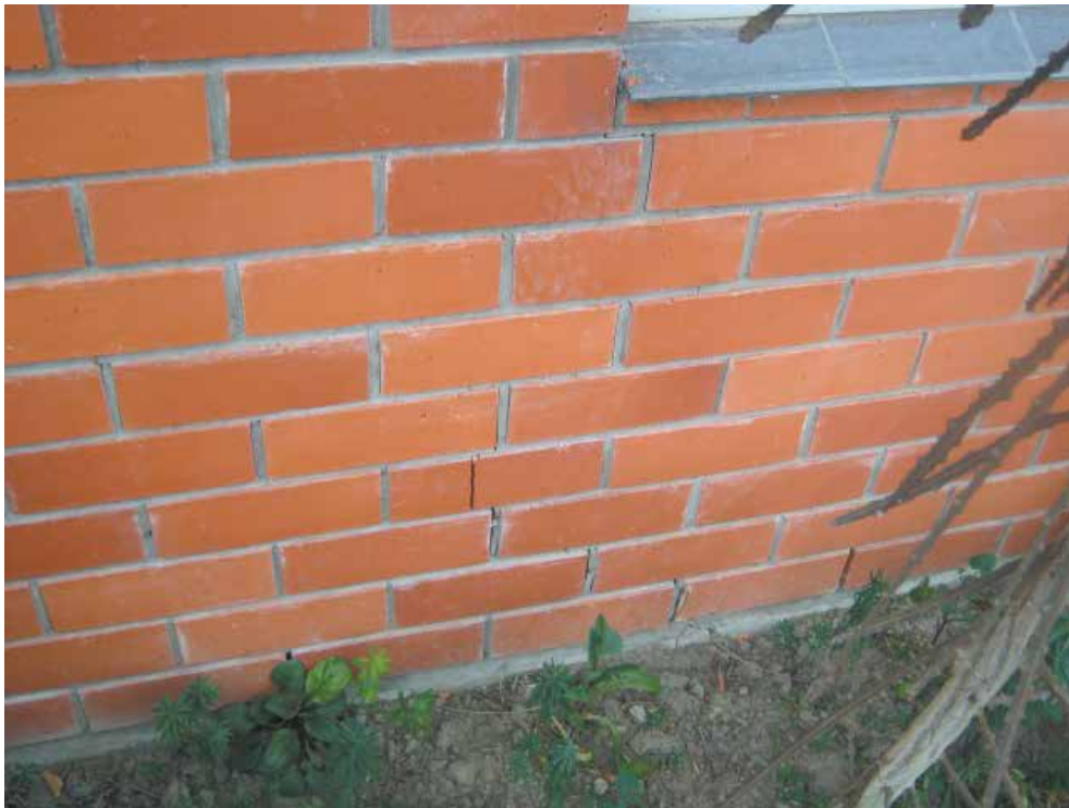
Image 1: Minor veneer damage, step cracking
