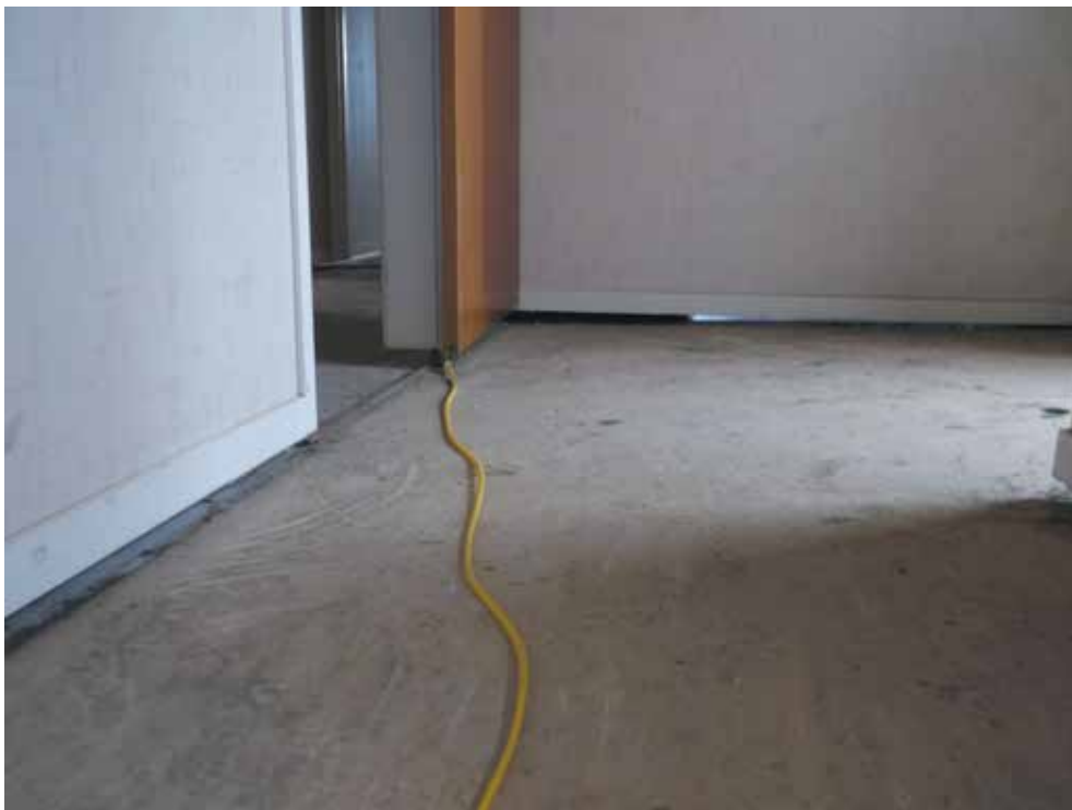
Image 10: Separation between slab and bottom plate was rectified by mechanically lifting centre of slab at several points. The slab then had the void filled
