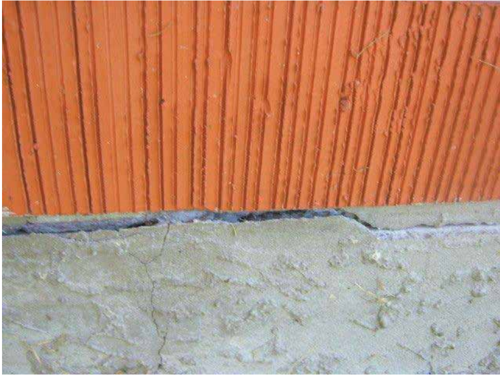
Image 2: Minor damage to perimeter foundation
