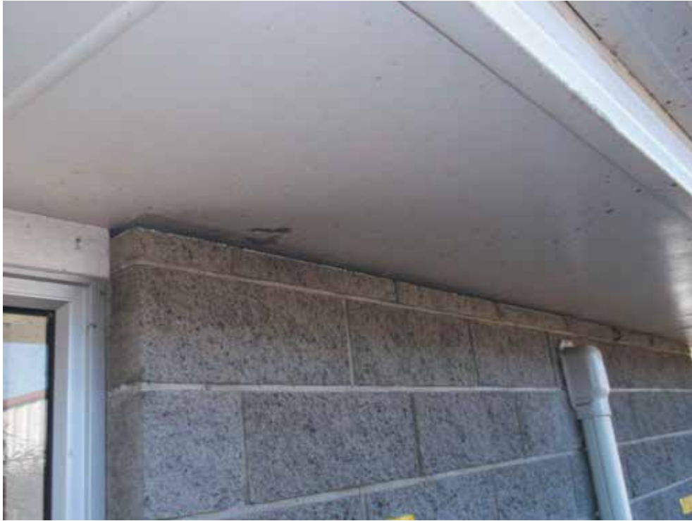
Image 10: Tapered gap between top of masonry veneer and soffit due to no structural connection between floor slab and foundation perimeter beam
