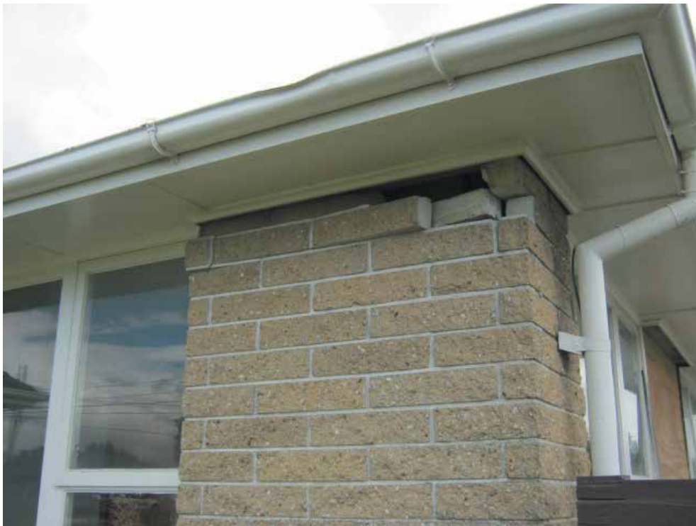
Image 1: Damage to brick veneer at soffit
