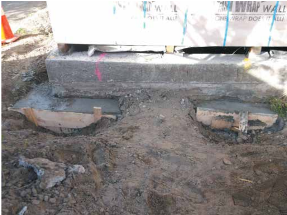
Image 9: Void fill under footing
