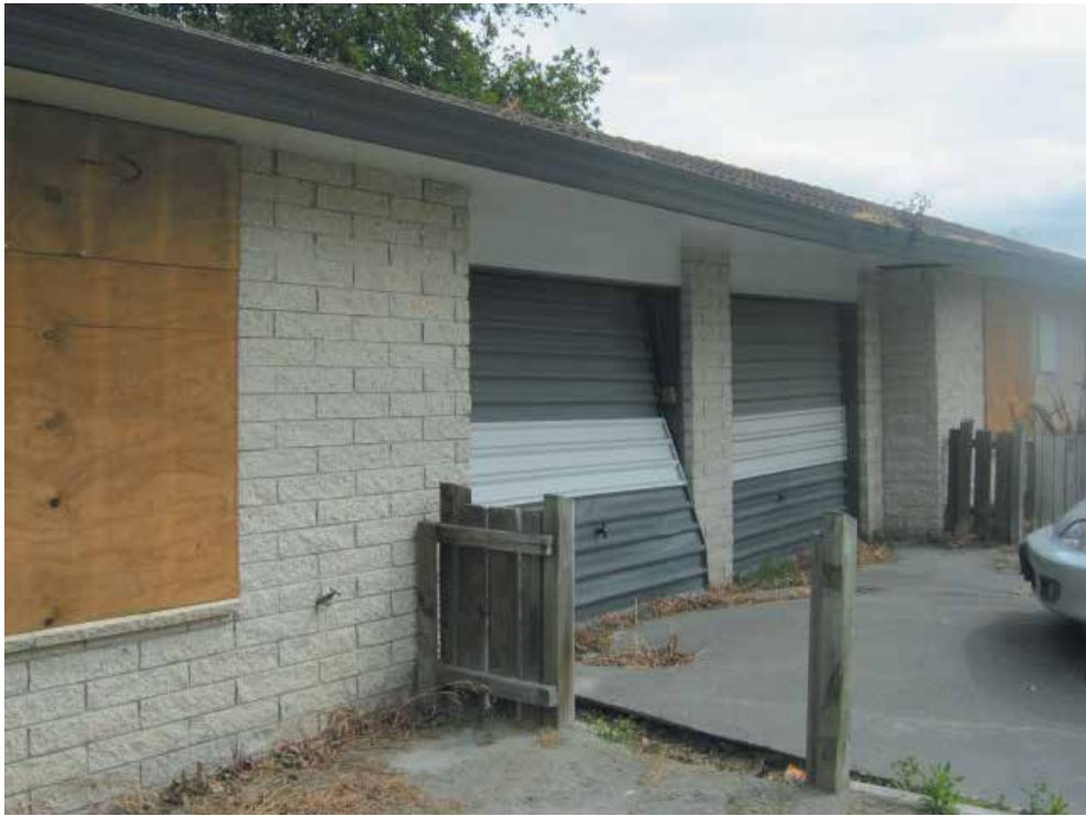
Image 2: Attached garages settled below driveway raised by liquefaction ejecta
