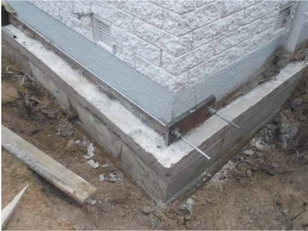
Image 11: Tension bars pulled foundation together closing up cracks
