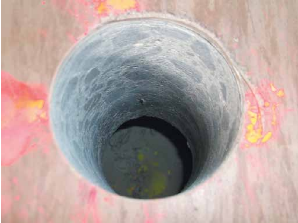
Image 8: Internal core holes drilled in slab for void fill injection points and internal mechanical lifting points
