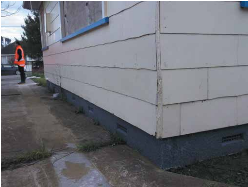
Image 1: No earthquake damage to exterior cladding
