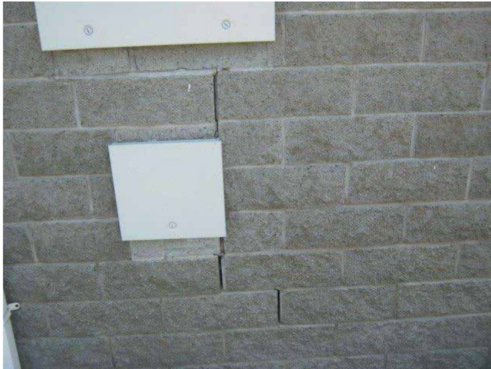
Image 2: Lateral spread of Summerhill Stone veneer cladding
