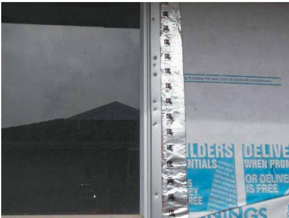
Image 11: New building wrap installed. 50x50mm flashings to windows to provide cover at window brick junction
