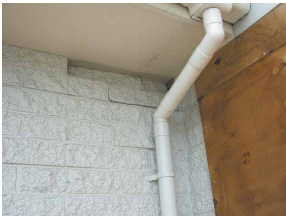
Image 1: Moderate damage to Summerhill Stone cladding
