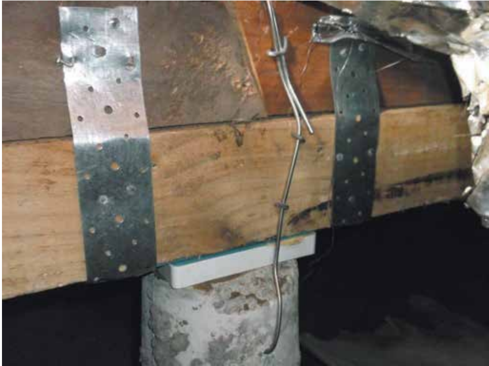
Image 10: Areas requiring over 100mm packing were jacked, packed and strapped using double bearers
