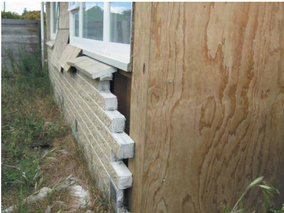
Image 3: Masonry veneer separated from structure
