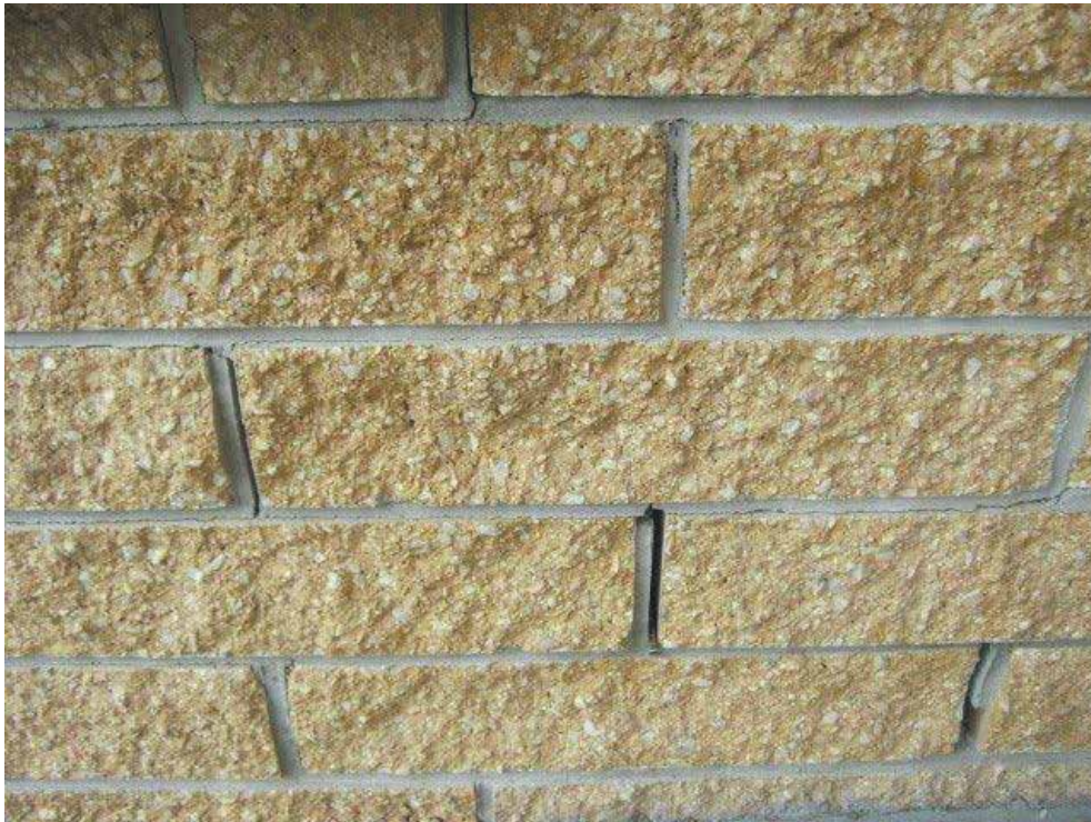
Image 1: Minor step cracking in veneer
