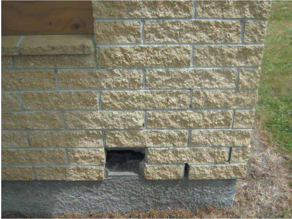
Image 2: Minor damage to brick veneer
