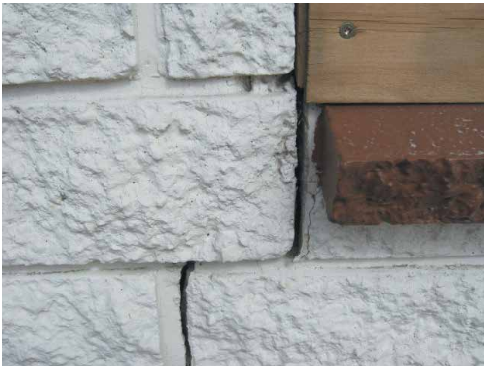
Image 3: Step cracking from openings caused by differential settlement of the foundation
